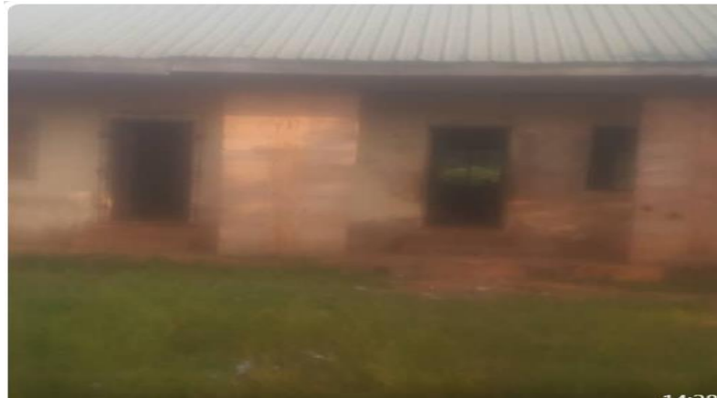
Figure 4:16: The image above depicts the lack of structural accessibility for children with physical disabilities.
