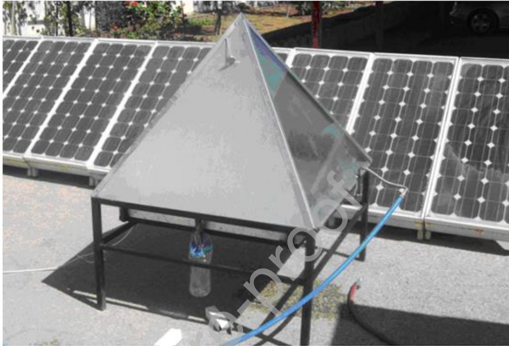
Fig. 4 Photograph of the solar distillation system integrated with photovoltaic (PV) panels
