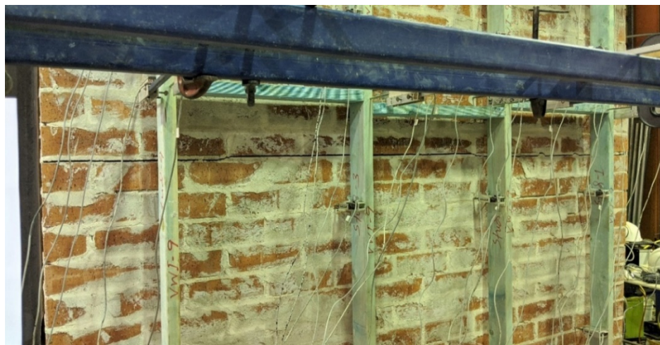
Figure 8: Brick Veneer Cracking Under Out-of-plane Loading
